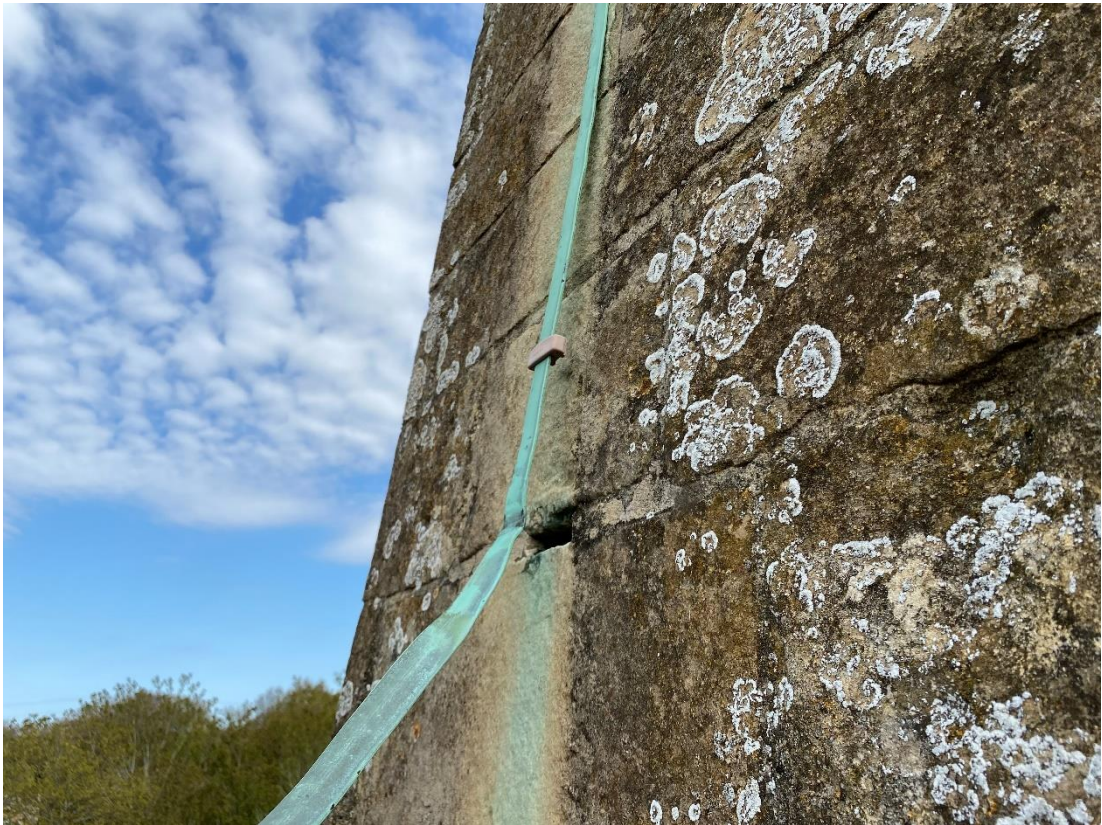
7.5 Spire lightning conductor
